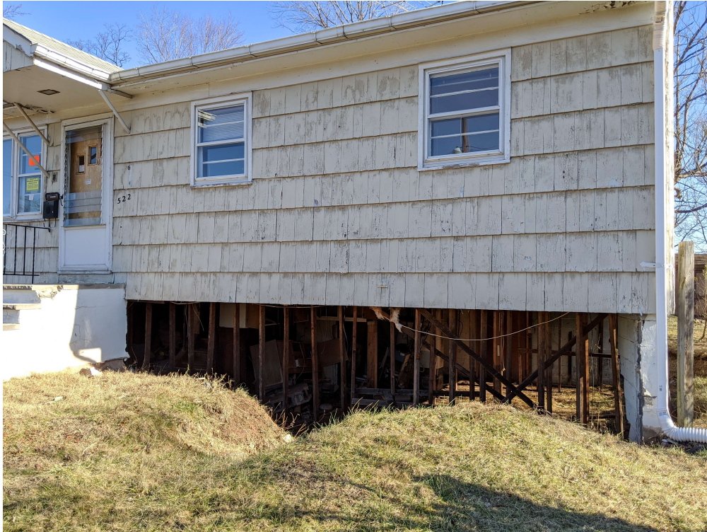
Signs outside this home in Woodbridge, N.J. say it is unlawful to inhabit. An exposed basement shows the remnants of flood damage.
